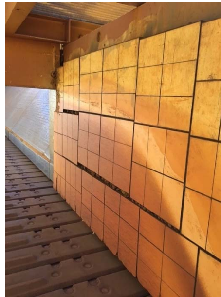
Photo 8 Magnetic Panels that have moved
