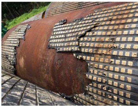
Figure 1 Debonding of the Lagging From the Pulley Shell
