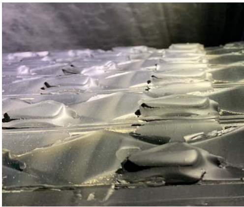
Figure 9 Pulley Lagging Failure in Drive 1
