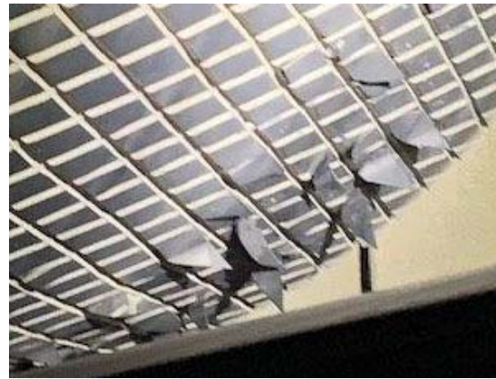
Figure 10 Pulley Lagging Failure in Drive 2
