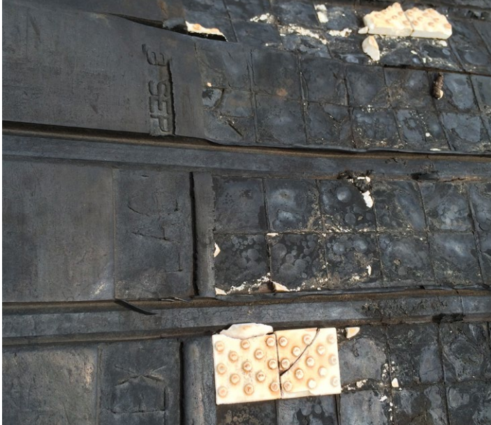
Ceramic tile loss due to debonding
