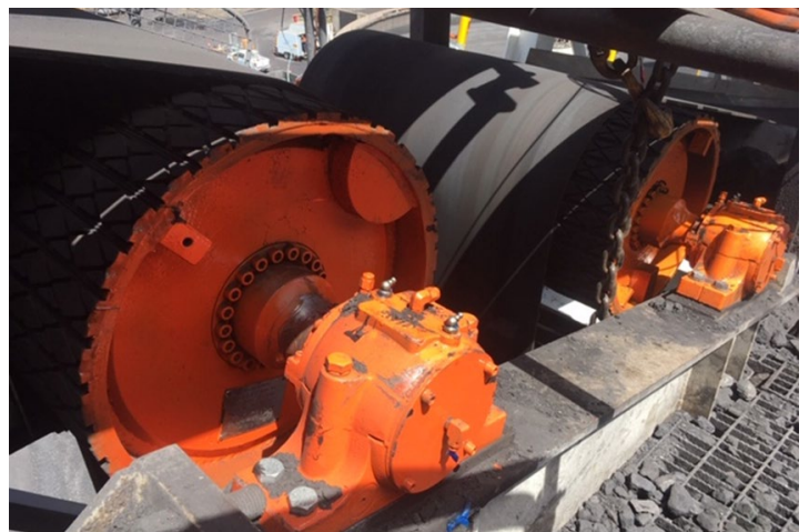
Elastotec HV FRAS Diamond Lagging Installed and operating at Curragh
