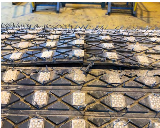
Photo #2. Cold vulcanised lagging failure due to debonding under load at low temperature.
