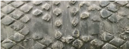
6MW Drive NSW, Australia, Melting of rubber
