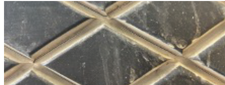
20MW, Copper, Chile. Rubber cracks inside grooves
